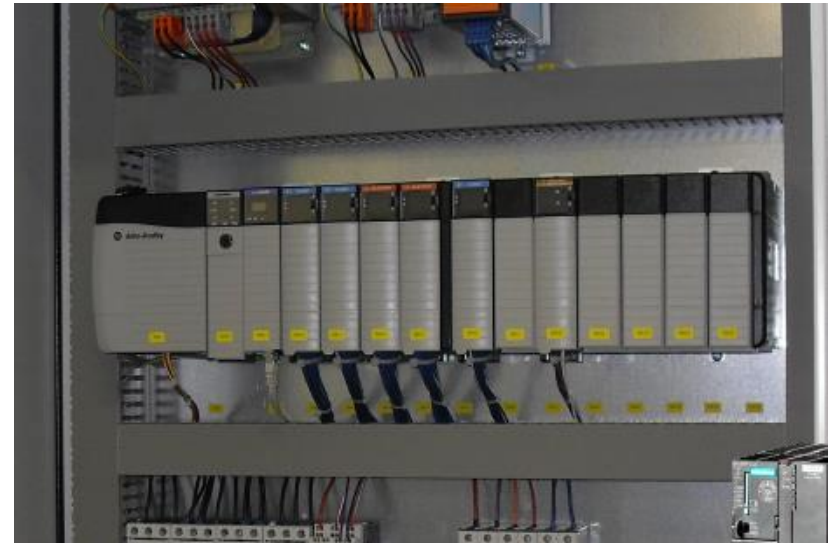
PLC – Programmable Logic Controller
